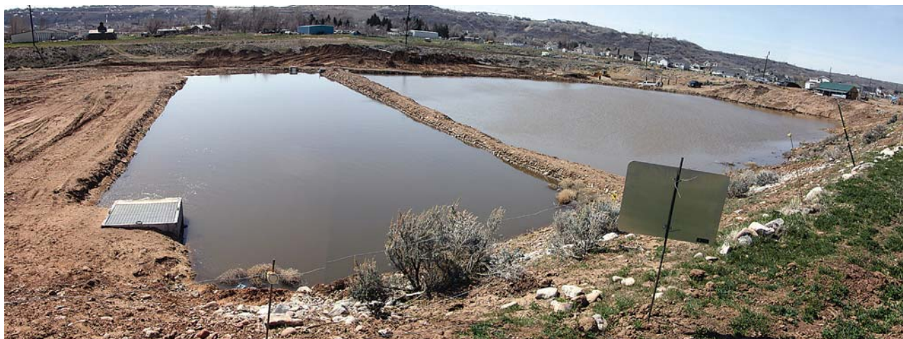
The Weber River Aquifer Storage and Recovery Pilot Project is located in a retired gravel pit near the mouth of Weber Canyon. Shown here are two of the project's four recharge basins filled with water in the spring of 2004.
