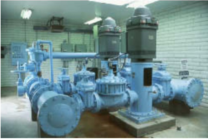
Where infiltration basins are not feasible, pumps can be used to inject water directly into the receiving aquifer. In some cases, the same pumps can also be used to recover the storage.
