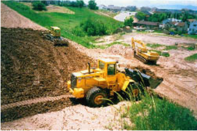
Water development will be needed to meet future demands. This development will be based on sound engineering, economic and environmental principles. (Photo of Adams Reservoir reconstruction near Kayville.)
